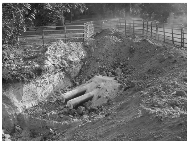
Heat plant distribution trench outside of Draper.
