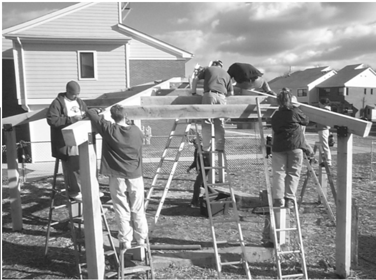
Students in Brad Christensen's TEC 107 (Residential Construction) class work on the frame for the solar shed. All lumber was milled from trees cut from the College forest.
